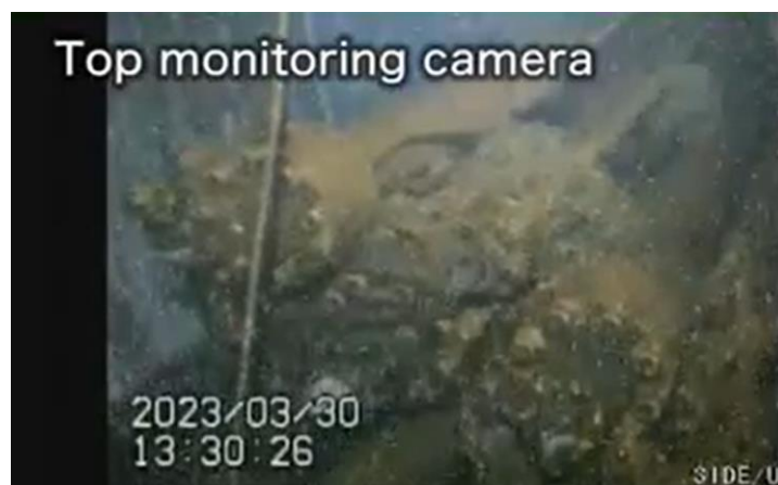
Figure 6-4: Dislocated CRD housings above the water level.
