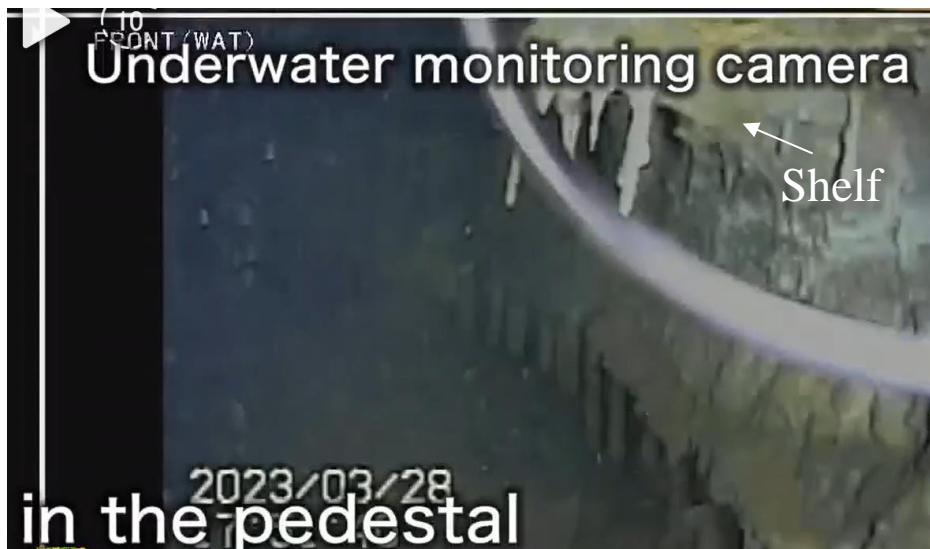
Figure 6-8: Protruding deposits above the concrete ablation area forming "shelf" structures.
