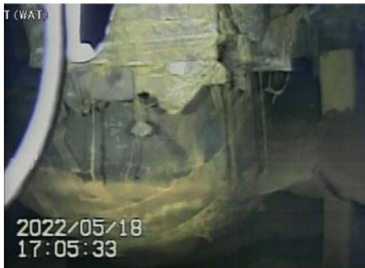
Figure 6-14: Damage on PLR piping.
