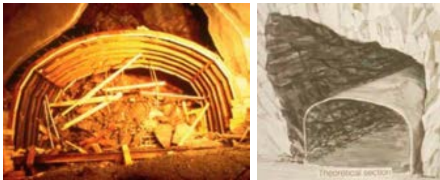
Figure 5: Photo and sketch of the overbreak experienced above the Forsmark 3 tunnel after intersecting the Singö deformation zone. From SKB R-07-10.
